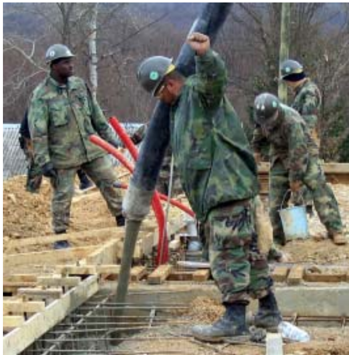
Humanitarian and civic assistance as part of a foreign internal defense program includes engineering construction projects.
